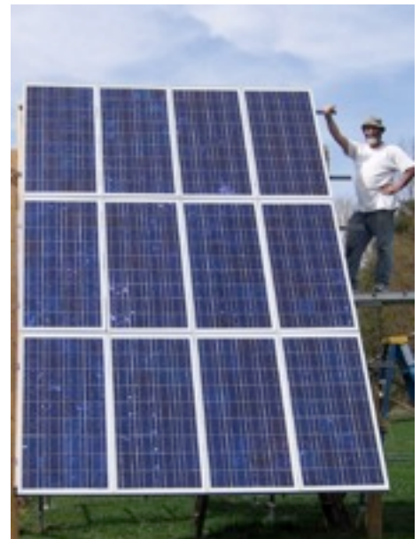
Photo-voltaic array (N1FMP)
